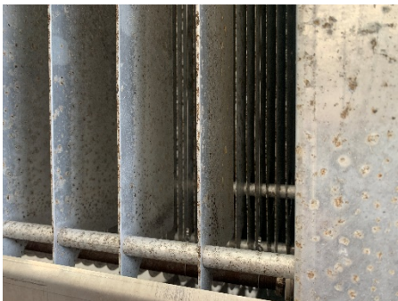
Low grade aluminium cell showing signs of rust in a RydAir unit (AOS Australia).
